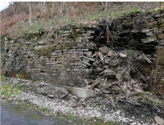
Figure 16 – wall in state of disrepair
